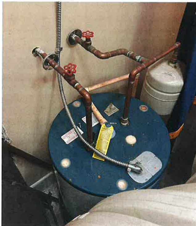
Existing 30-Gallon Electric Tank Water Heater (Second-Floor Storage)
